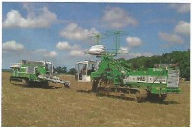
Miles Drainage provides a GPS based land drainage design and installation service nationwide.
