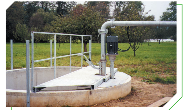
Permanently installed LE model used for transfer
