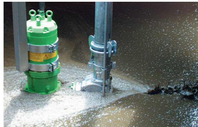
Feeding of the system with a special submersible motor chopper pump
